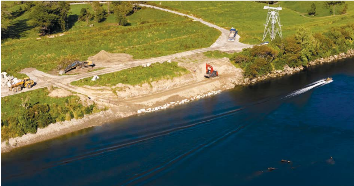
Stopbanks under construction on the Buller River as it flows past Westport to meet the Tasman Sea. Photo / AG Images
